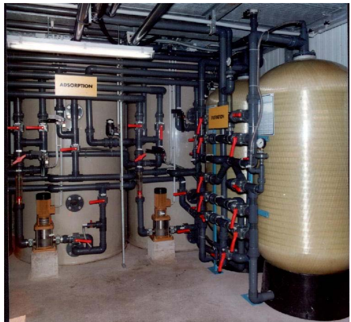
View of the filtration and adsorption treatment stages in the ground floor.
